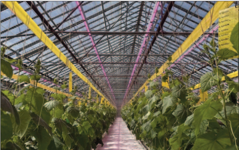
Recently installed LED lighting helps maintain crop performance through shorter winter days.
