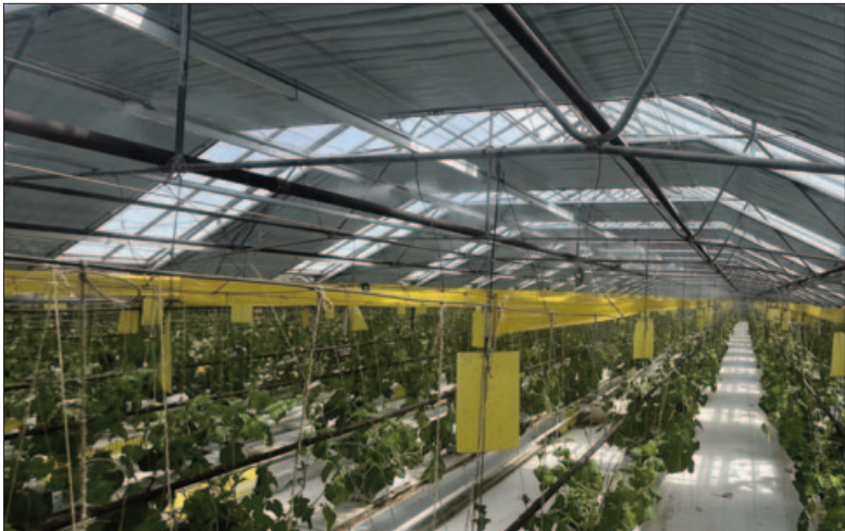
New automated energy curtains improve energy efficiency while enhancing growing conditions in older greenhouse structures.
